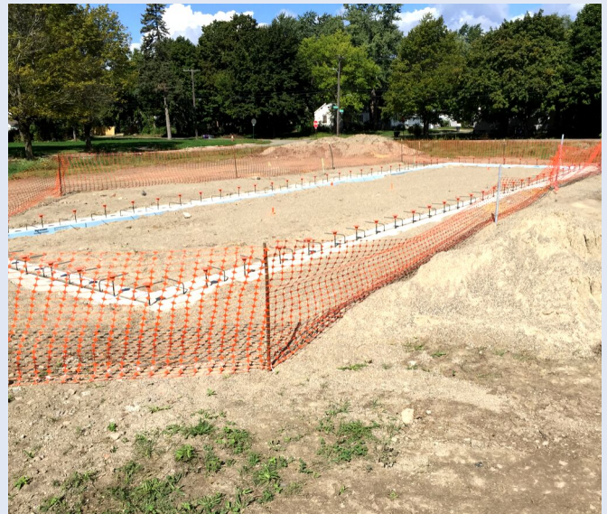
Above: The footing for the foundation of the first building at the DPFLI.
