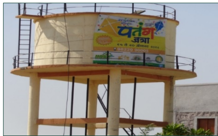
Figure 17-5. Overhead tank for water supply at Palshi.
