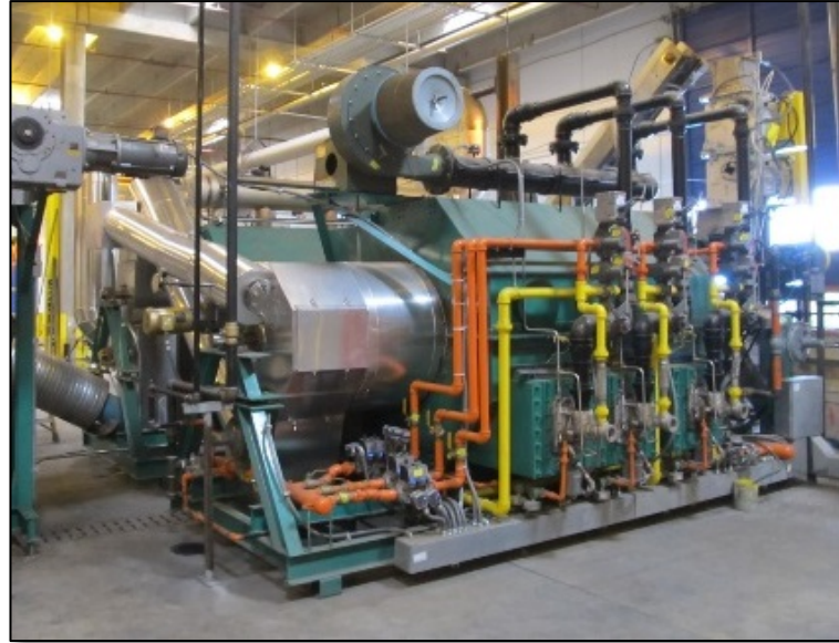
Tucker RNG biomass gasification system developed in partnership with USFS.
