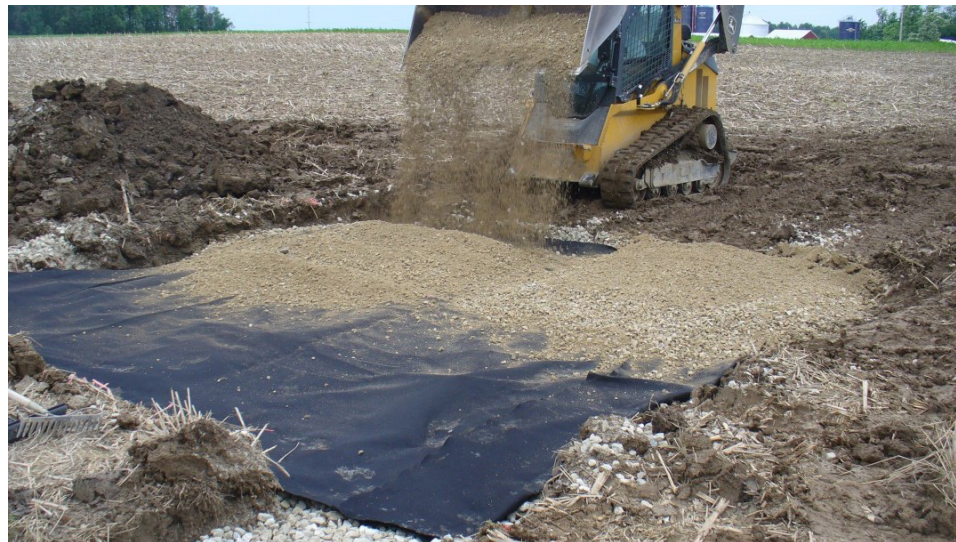
Figure 4- Top: Coarse gravel being poured over the perforated collection pipe. Bottom: Sand being poured over the nonwoven geotextile fabric (photo credit: Justin L. McBride).
