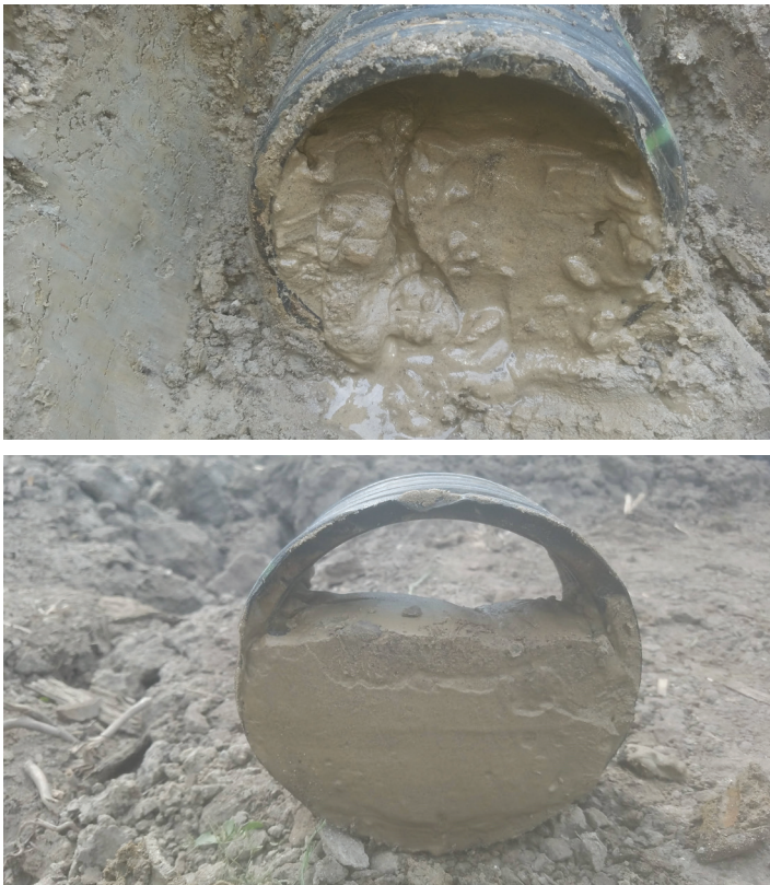
Figure 2- A 6-inch main, installed in 2013. The pipe was 2/3 filled with sand in 2020. The use of a regular-perforated pipe without a knitted-sock envelope in sandy loam soil was the cause of the drain sedimentation (photo credit: William Word).
