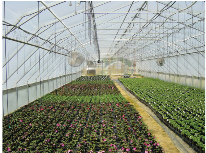
Figure 9. Horizontal airflow fans (HAFs) installed in a greenhouse to increase the uniformity of growing conditions. Photo courtesy of A. J. Both, Rutgers University.
