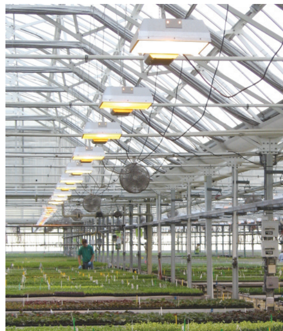
Figure 2. The high-pressure sodium lamp is still the most economical lamp type for most greenhouse supplemental lighting applications. Photo courtesy of Erik Runkle, Michigan State University.
