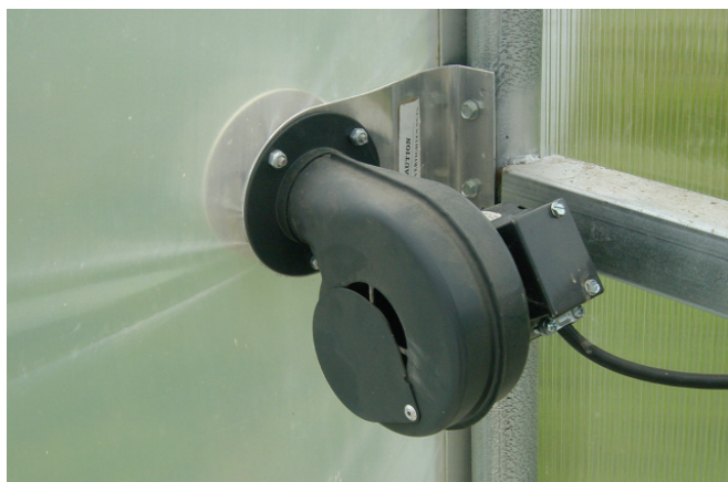
Figure 5. Since the air space between two layers of polyethylene provides insulation, the fans that keep the layers inflated should be routinely checked to ensure they are operating properly. Note that this fan is installed improperly: it should be pulling in air from the outside instead of from the inside of the greenhouse to reduce the potential for humid air causing condensation between layers. Photo courtesy of A. J. Both, Rutgers University.
