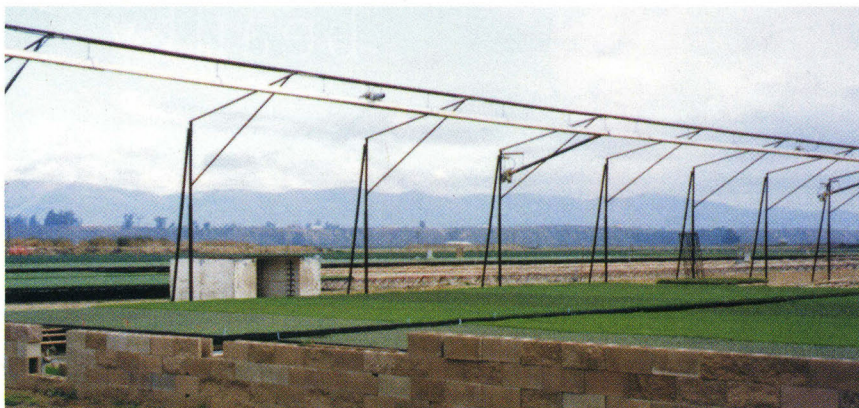
Hanging 16 feet above these 32-foot-wide beds, the infrared heating system has protected seedlings from frost when outside temperatures dipped to 14°F.
