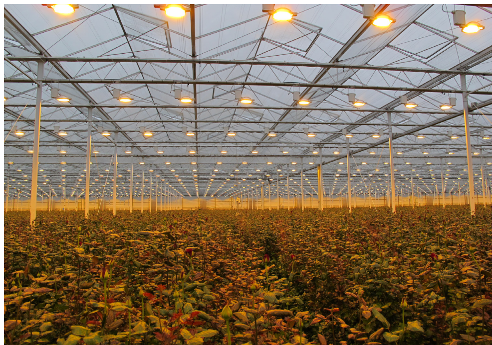
Fig. 1. Greenhouse supplemental lighting of rose cut flowers with high-pressure sodium (HPS) lamps
