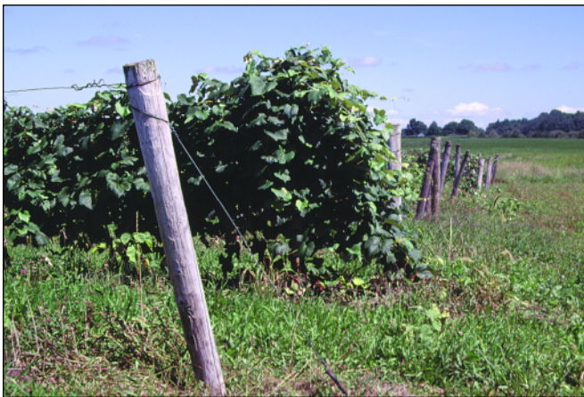
Fig. 27. The end posts in this vineyard were not adequately anchored. They have moved after installation to become this random arrangement.
