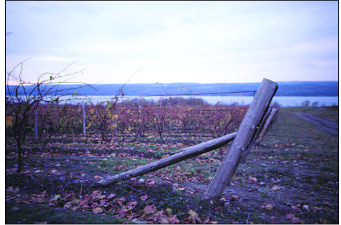
Fig. 30. Bracing an end post. This avoids conflict between equipment and external anchors in headlands but is more difficult and costly to install.
