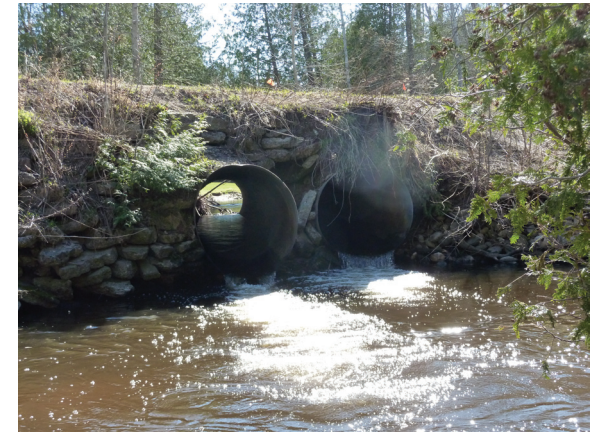
Photo 4-5: An old road crossing of a river that prevented fish passage and allowed sediment to pollute the river.
