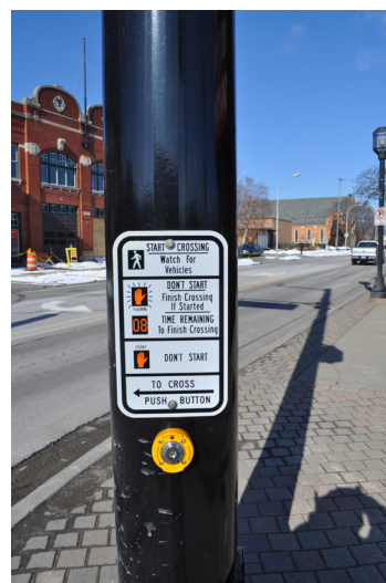
Figure 3.17, Pedestrian Actuated Crosswalk Signal
