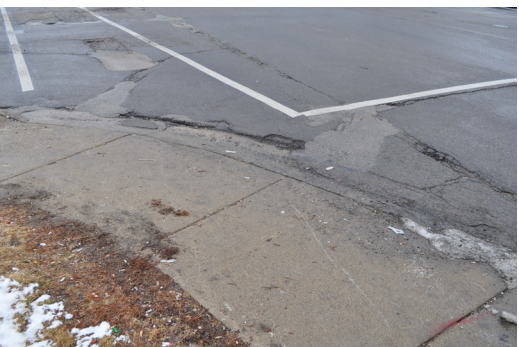
Figure 3.7 Missing Tactile Strips
