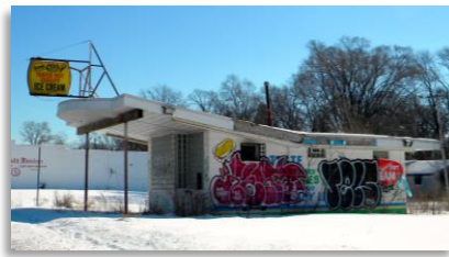
Figures 2.3.2, 2.3.3, 2.3.4 – Abandoned property within Focus Area Source: Practicum Team
