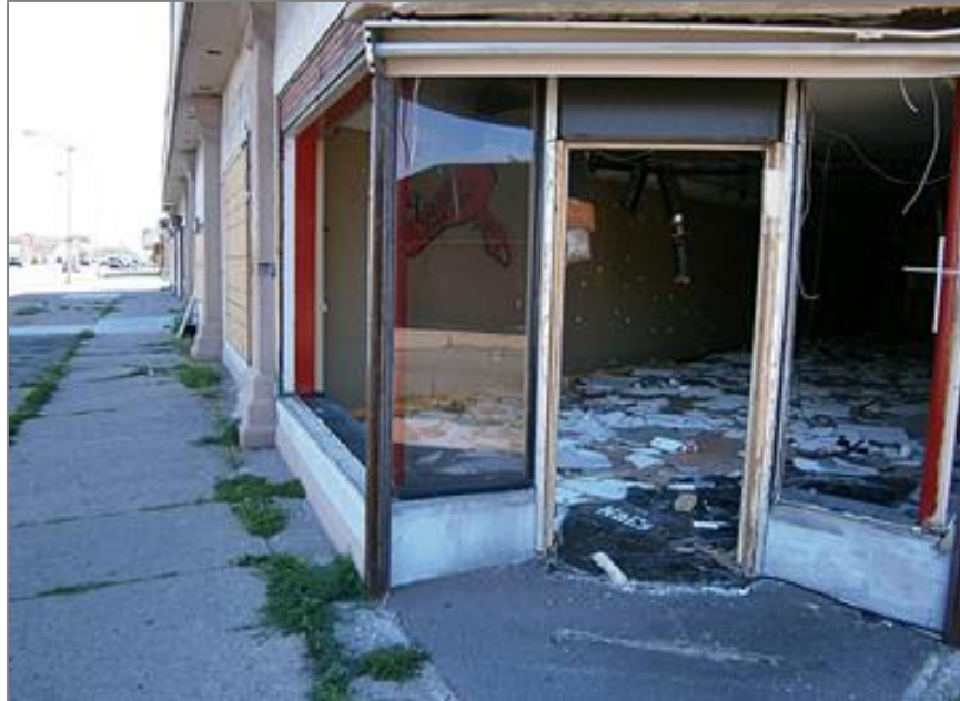
Figure 4.2.4.1 – Structure in ‘Complete Disrepair’ Example Source: http://ratkov.com/yahoo_site_admin/assets/images/Gratiot_july_112012_ret.272105344_std.jpg
