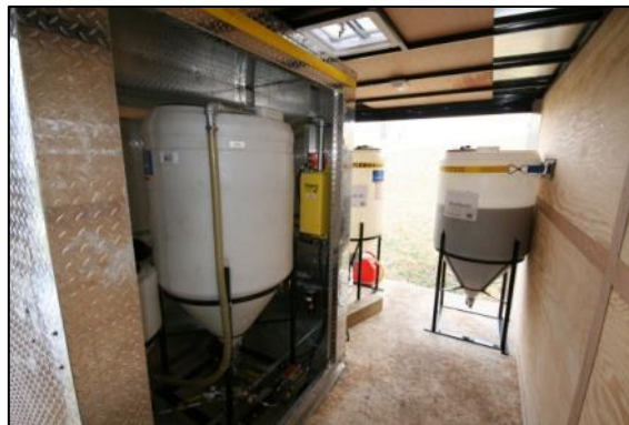
Biodiesel unit and storage tanks mounted inside enclosed cargo trailer.
