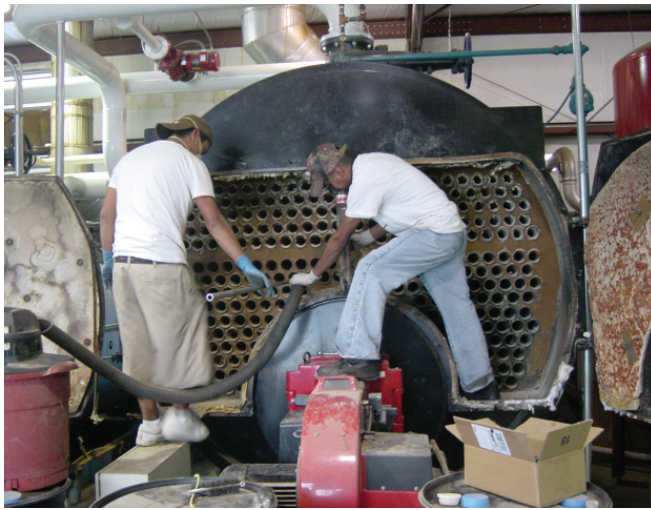
Figure 8. Regular boiler maintenance ensures proper operation and increases reliability of the heating system. Photo courtesy A. J. Both, Rutgers University.
