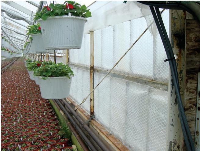
Figure 6. Plastic bubble wrap installed on the inside of the north-facing sidewall. The bubble wrap adds insulation but allows some light to enter the greenhouse through this sidewall. Photo courtesy of A. J. Both, Rutgers University.
