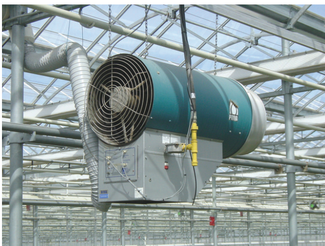
Figure 7. Gas-fired unit heater installed in a greenhouse to deliver hot air. Photo courtesy of A. J. Both, Rutgers University.
