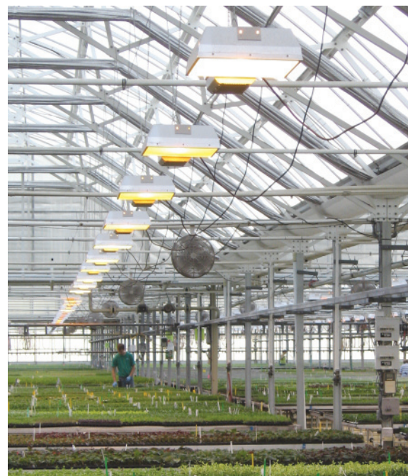
Figure 2. The high-pressure sodium lamp is still the most economical lamp type for most greenhouse supplemental lighting applications. Photo courtesy of Erik Runkle, Michigan State University.
