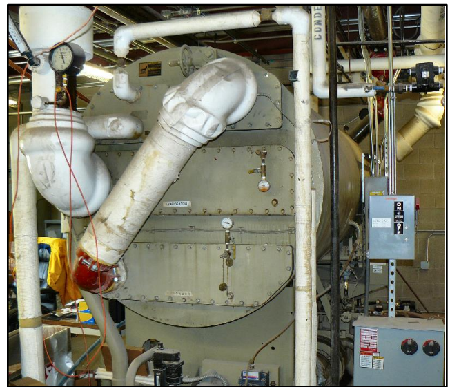
Above: Absorption chiller.
