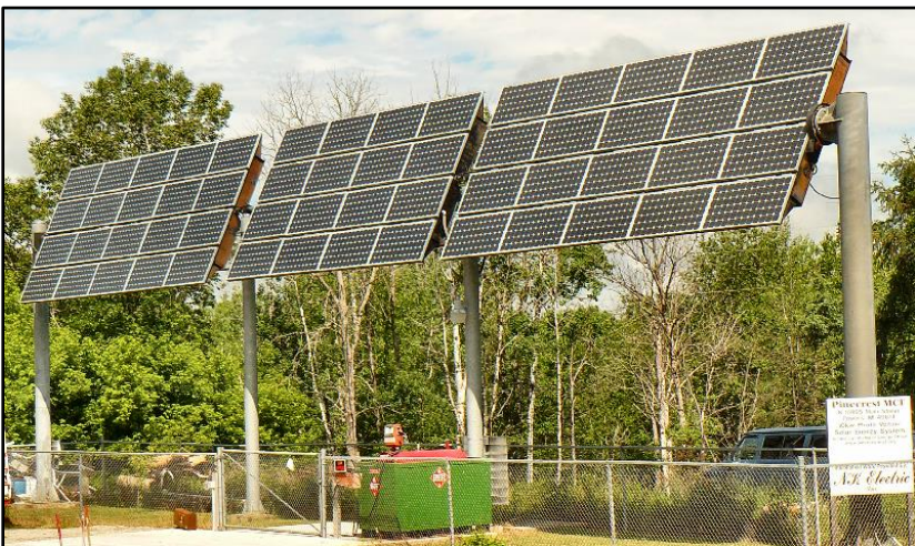
Below: 10kW solar array.
